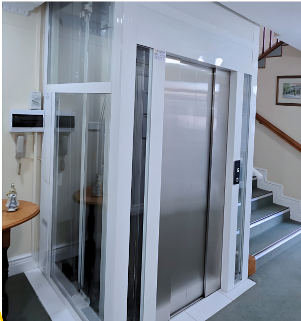
RETIREMENT VILLAGE, KZN Description: 1 Home Lift
