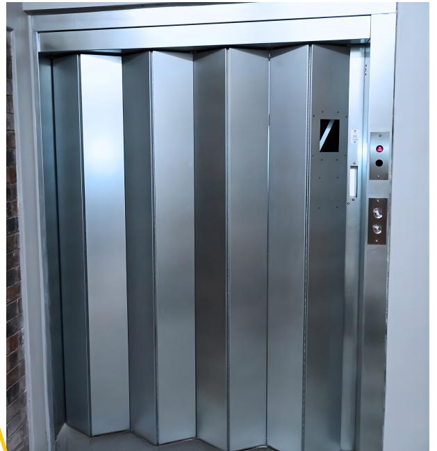
SHOPRITE, MERRYDALE JUNCTION Description: 1 Goods Only Hoist
