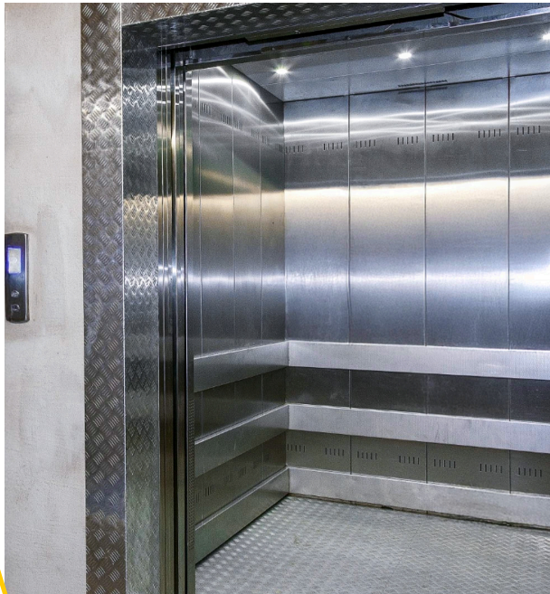
BALLITO MALL • Client: Flanagan and Gerard / Menlyn Maine Description: 7 Passenger Lifts, 10 Goods Lifts and 4 Goods Only Hoists
