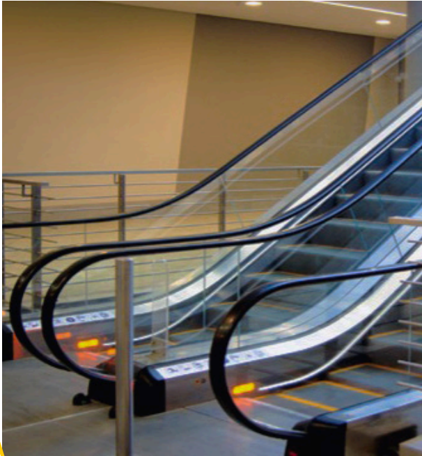
CORNUBIA MALL • Client: Investec Property (Pty) Ltd Description: 12 Escalators
