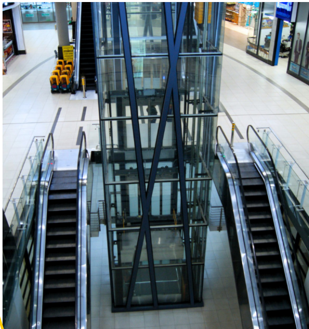
WATERCREST MALL • Client: Acucap Properties Description: 5 Passenger Lifts and 3 Goods Lifts
